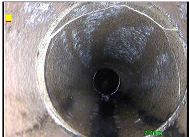
MH2X_1e8c07a4-1196-4862-93c4-2a00363de73a_20190719_091217_436.jpg, 00:00:42, 7.41 m Cracks, multiple from 12 o'clock to 12 o'clock
