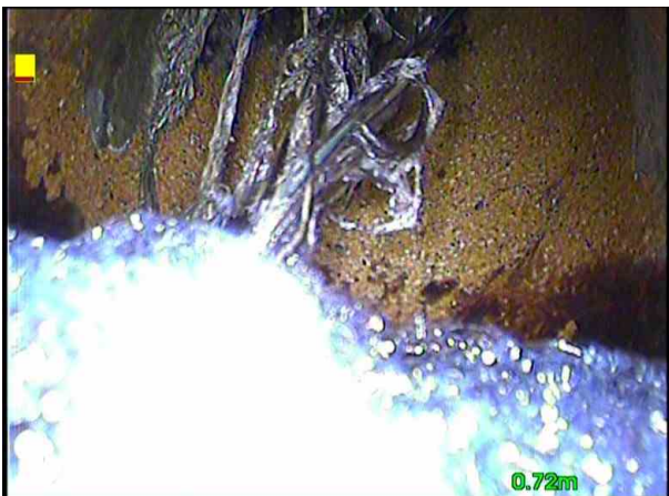
WCX_ea51cb9a-adf6-4fb3-9f3d-a36a19991198_20190719_092201_694.jpg, 00:00:15, 0.73 m Other obstacles, other object in invert at joint from 12 o'clock to
