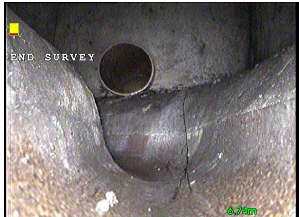
MH1X_688e7929-c132-4a3d-9f6a-1c4287db6ddd_20190719_090729_862.jpg, 00:00:00, 6.74 m Finish node type, manhole, reference number: MH1
