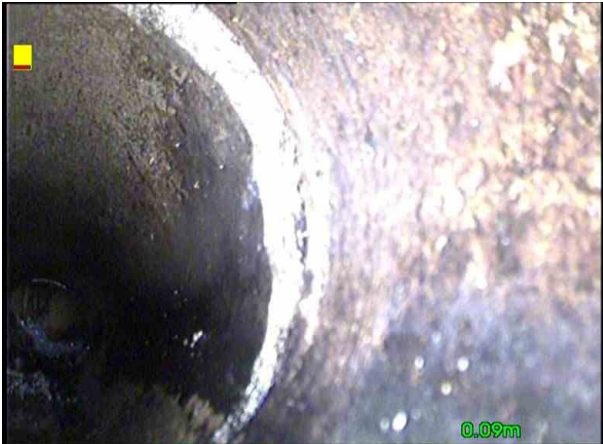
WCX_db63b882-4aba-429c-9ff7-fb83d9a492a5_20190719_091904_894.jpg, 00:00:06, 0.09 m Joint displaced, medium
