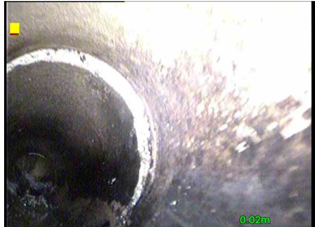
WCX_c514130f-8838-4540-ab91-79de0b5f209d_20190719_091915_100.jpg, 00:00:06, 0.09 m Joint displaced, medium
