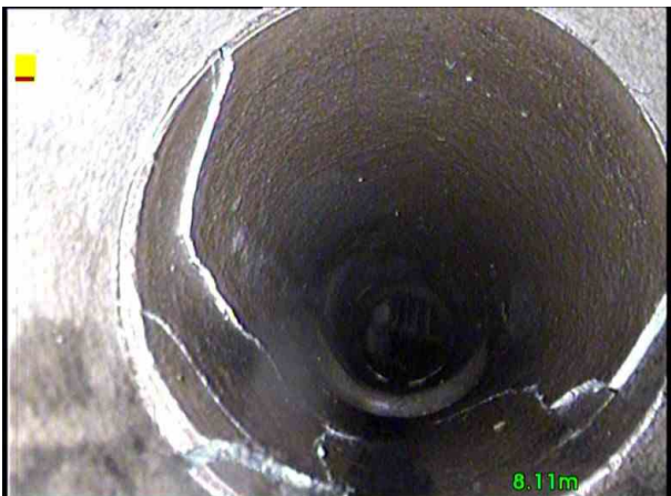
MH2X_0cb3d7ea-633a-47b0-9714-cf7fc0eb537a_20190719_091240_738.jpg, 00:00:46, 8.11 m Fractures, multiple from 12 o'clock to 12 o'clock
