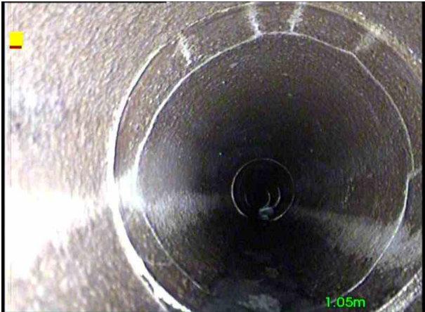
MH2X_d1f88f49-95b6-4301-a031-a1a0e0d241b7_20190719_090934_524.jpg, 00:00:13, 1.05 m Cracks, multiple from 12 o'clock to 12 o'clock
