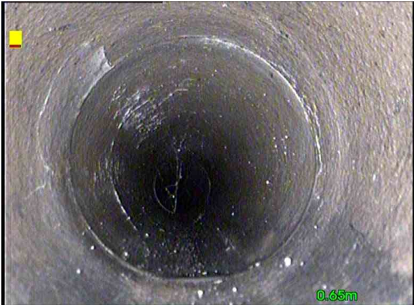
MH1X_02ace76e-24f9-408b-a62d-7bff35a29c37_20190719_090353_612.jpg, 00:00:16, 0.65 m Crack, circumferential from 12 o'clock to 12 o'clock
