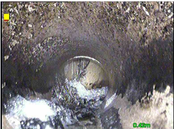
WCX_103231f6-ffab-4e4a-bacb-05face603c94_20190719_092045_737.jpg, 00:00:10, 0.44 m Other obstacles, other object in invert at joint from 4 o'clock to
