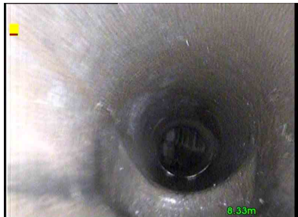
MH2X_9a43973b-9cd2-4c72-acdc-7cb9bfae800b_20190719_091347_476.jpg, 00:00:51, 8.42 m Junction at 6 o'clock, diameter: 150mm, BACKDROP
