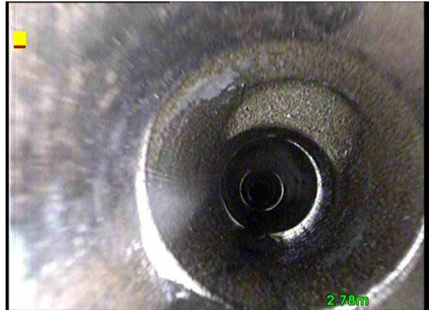
MH2X_9e4c6c1b-8d0a-40b1-b85c-89186ece19ae_20190719_091020_444.jpg, 00:00:22, 2.78 m Joint displaced, medium
