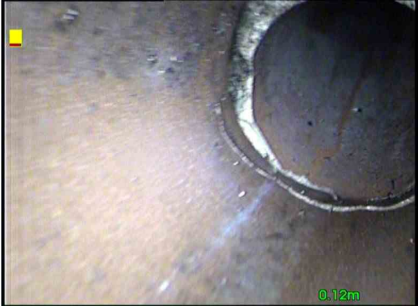
GULLYX_ea12e868-f5db-475e-aeac-0d1df9fea055_20190719_091651_803.jpg, 00:00:08, 0.28 m Joint displaced, medium
