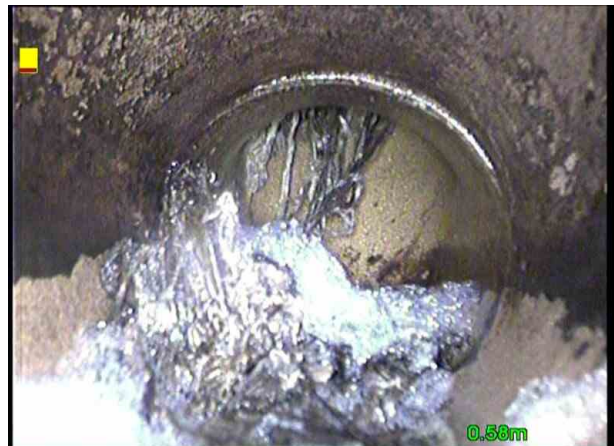
WCX_c872ec96-1e5d-438a-8b45-e22b98e4de62_20190719_092051_635.jpg, 00:00:10, 0.44 m Other obstacles, other object in invert at joint from 4 o'clock to
